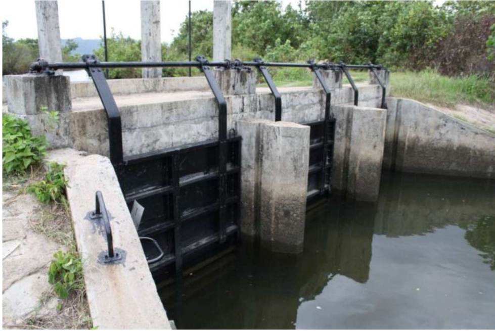
Figure 3. One of the outlet structures of the Prey Nub Polders. At the polder side vertical gates and at the sea side flap gates (locally called baffles) (Emmerik and Piet, 2012)
