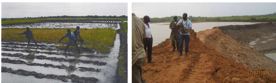
Tillage in a paddy field with two previously treated Periques in the background ( Vakgroep Weg- en Waterbouwkunde en Irrigatie , 1988) and construction of a dam in a creek
