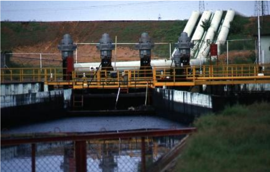
Figure 2. Electric drainage pumping station and the dike of Polder Lagunillas, one of the Bolivar Coast Polders
